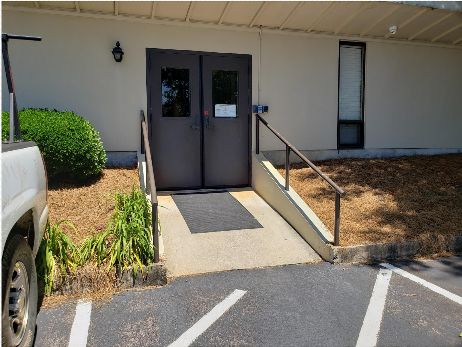
new landing, stairs, ada ramp, and covered entryway at grace center rear doors
